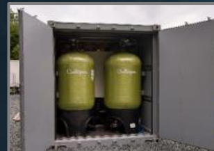
Granular Activated Carbon Vessels
